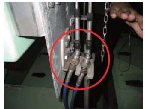
Release cable bent
