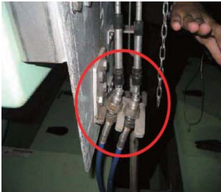
Defective release cable
